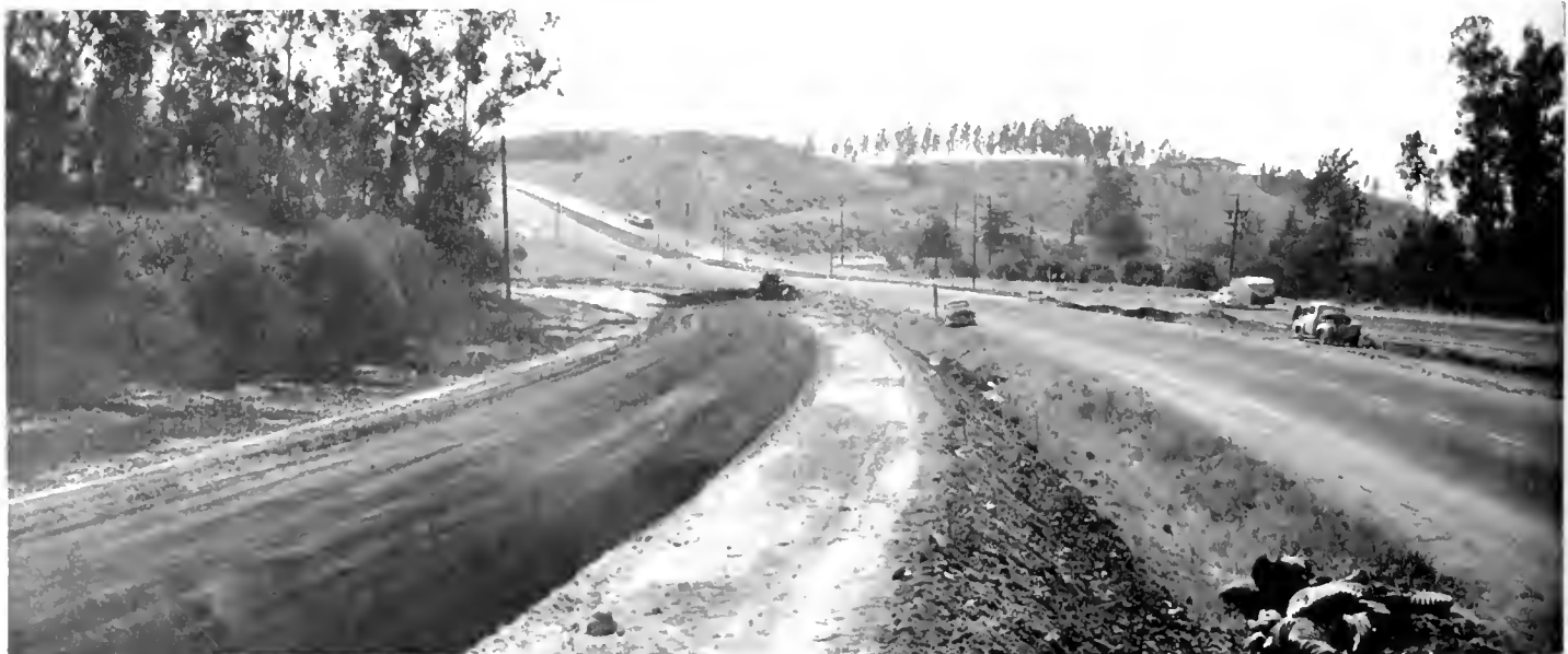
At easterly terminus of contract looking southerly on Route 43 at temporary connection for detour to new frontage road
